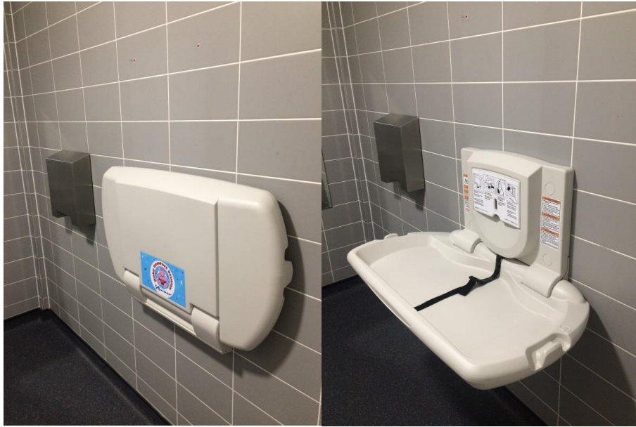
Figure 68:Baby changing facilities installed in both male and female Biosciences rest rooms. Currently nursing facilities are available in the adjacent Medical School. As the department grows further we will review having our own facilities (Action 5.11).
